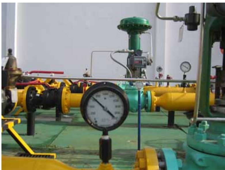
Flow measuring post for natural gas in Bolivia
